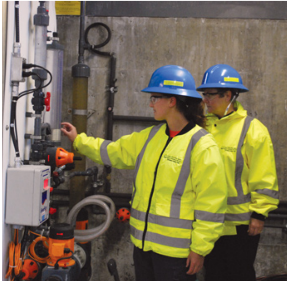
Operator Mandi Larose and PCT Debbie Turner inspecting aluminum sulphate chemical feed panel
