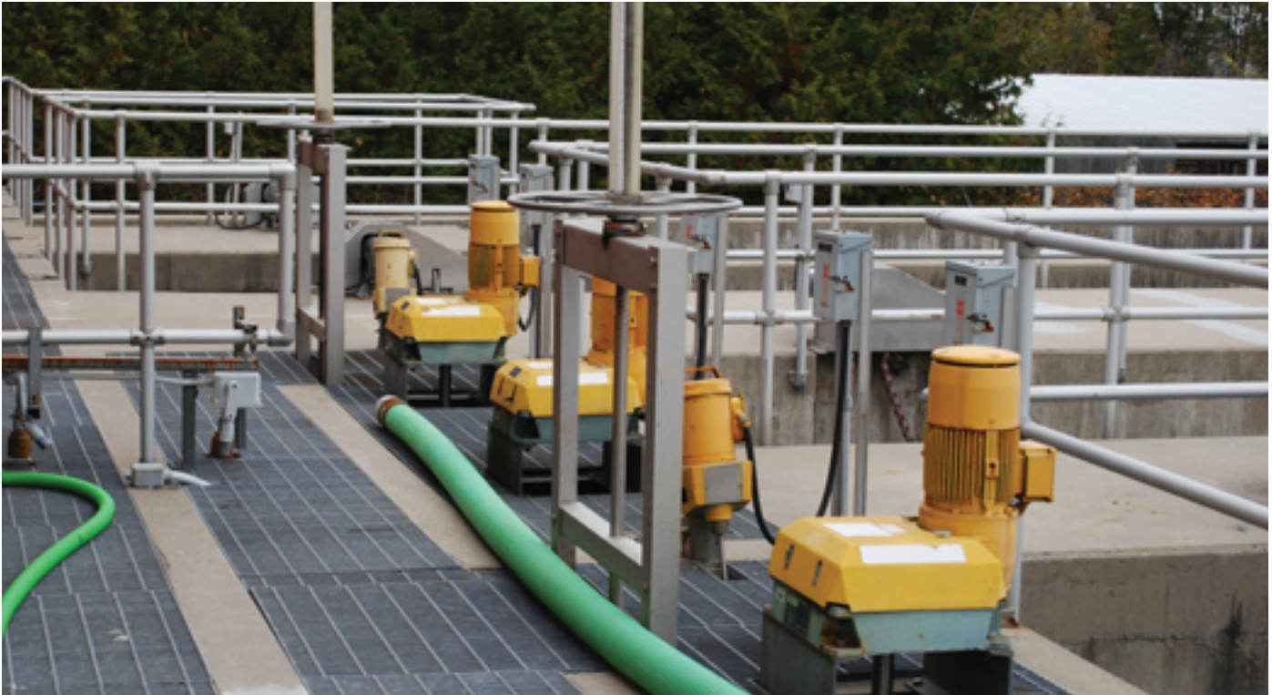
WWTP primary clarifiers and process mixers used during high flow events – ready for action
